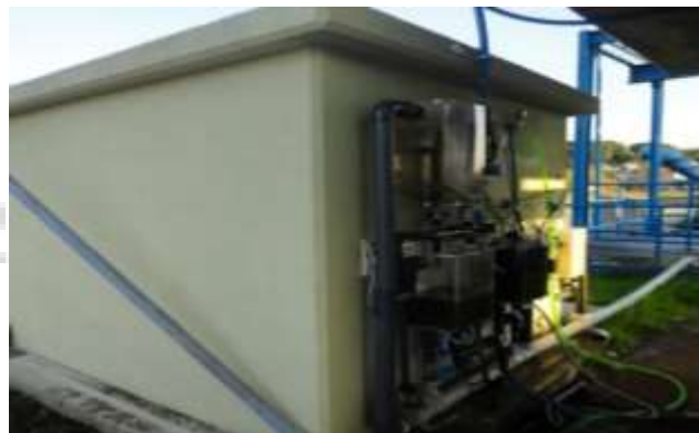
Figure 5: Aboveground mansion wastewater and clean water connections
